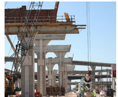
Here is a picture of the current progress on the supports for part of the interchange.
